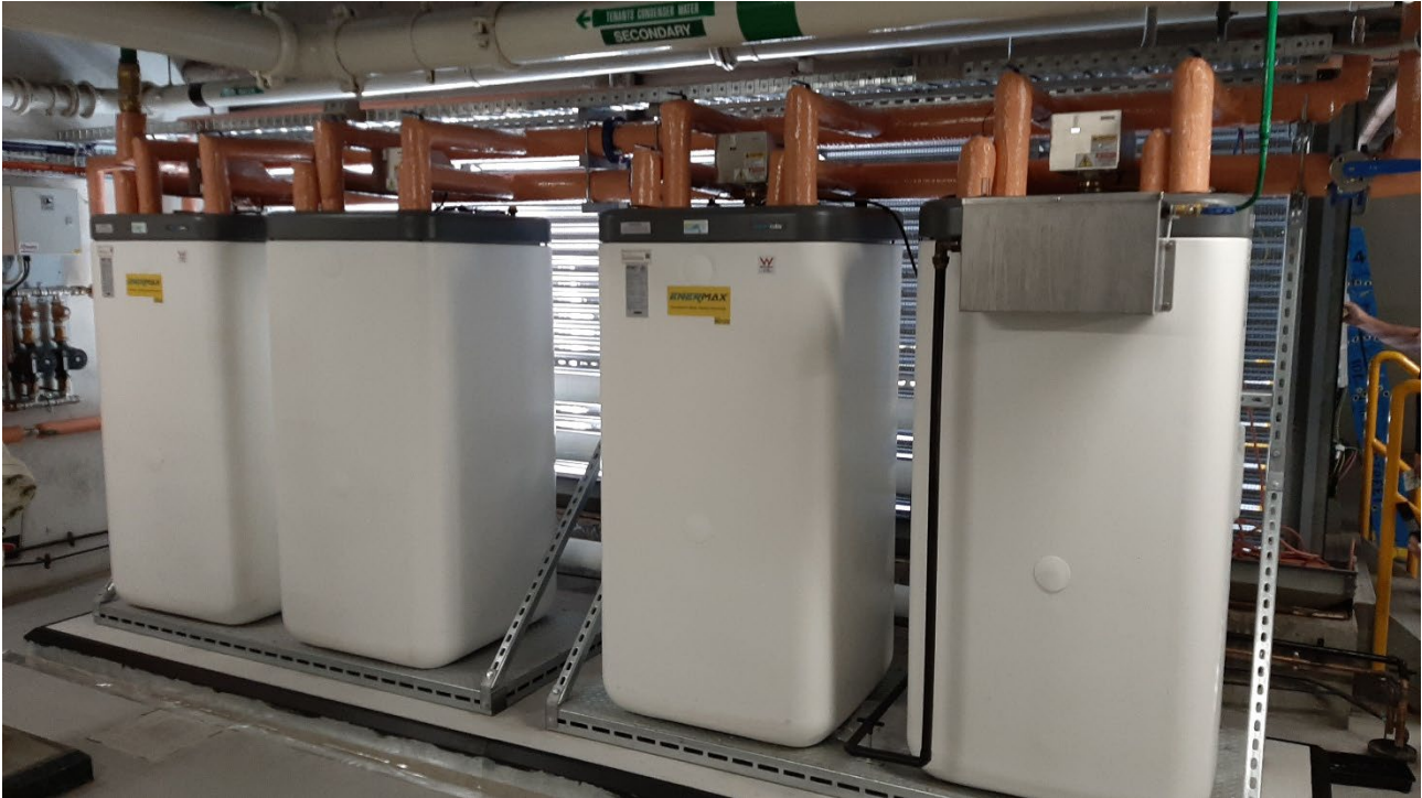
Figure 15. Insulated thermal storage tanks in a Melbourne office building. Source: Energy Smart Water.
