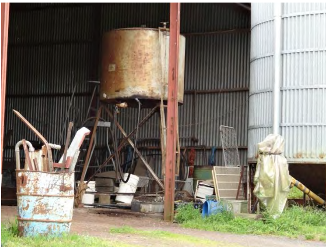
Plate 7.7 : Above ground diesel storage tank at property 6
