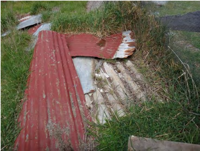
Plate 7.5 : Potential asbestos cement sheet at property 2
