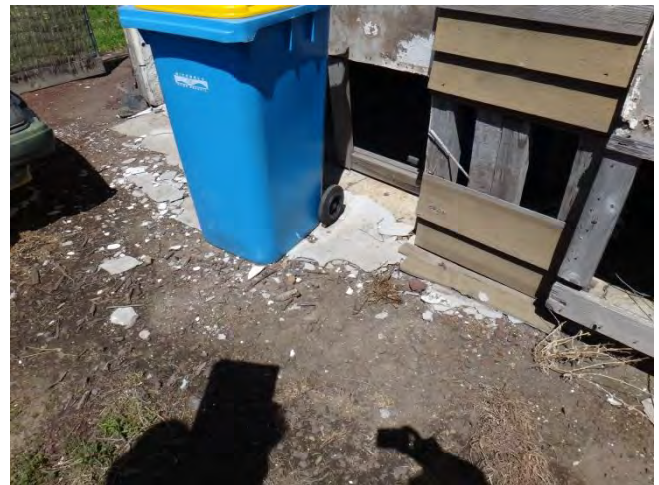
Plate 7.8 : Potential asbestos cement sheet at property 22
