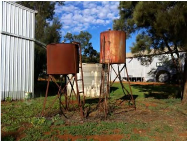
Plate 7.1 : Example of above ground storage tank
