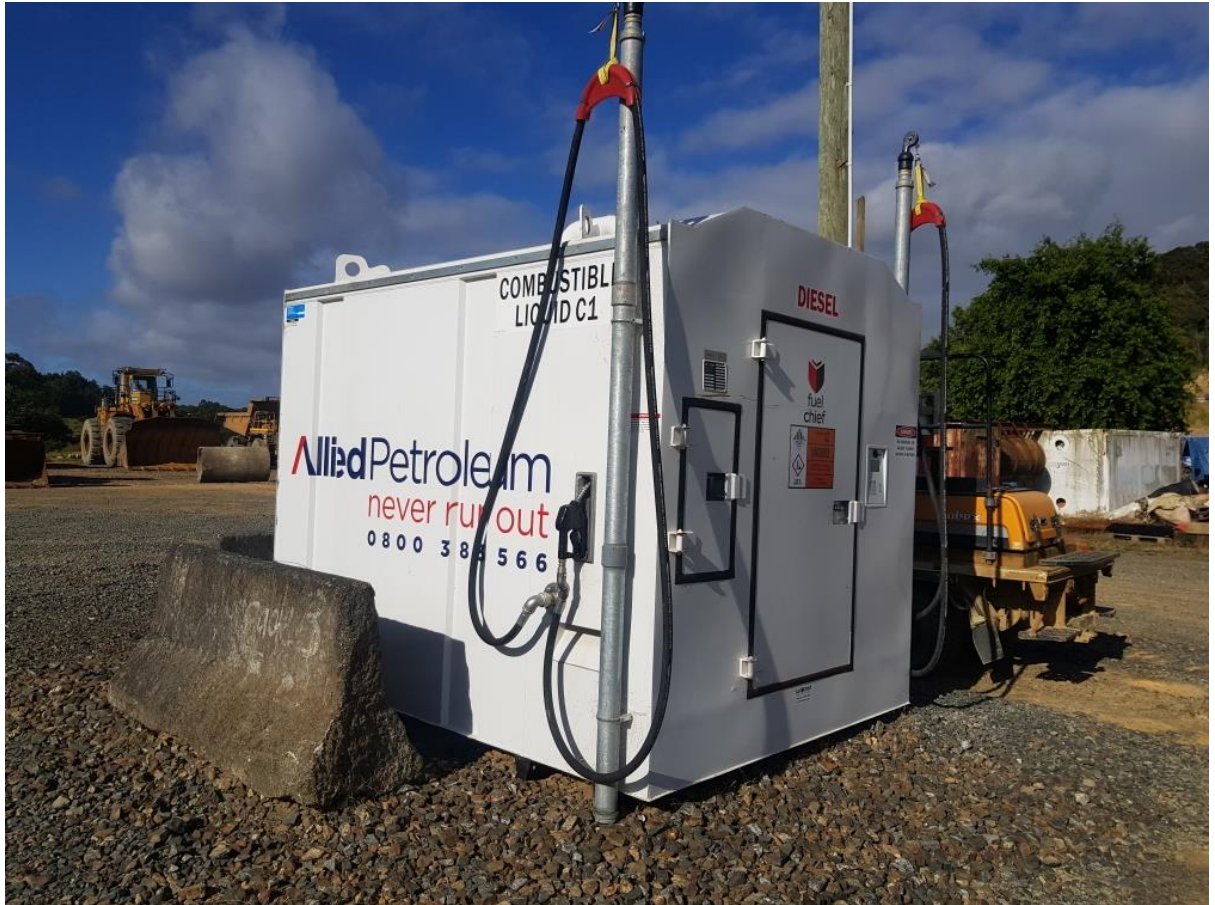
FIGURE 1: Fuel Storage Tank 7
