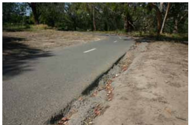
Figure 16 – Longitudinal cracks near the edge of a path can also be hazardous to cyclists.
