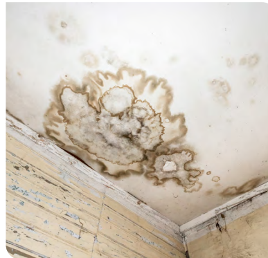
Mould spots on ceiling or floor
