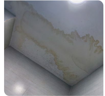
Water stain on ceiling
