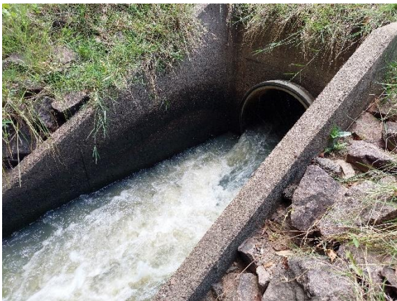
Photo 23. Piped culvert under a farm road crossing of the Didgeridoo Lagoon system drainage channel just upstream of its confluence with East Barratta Creek. High flow velocities and vertical drops create a fish passage barrier that could only be circumvented during flood inundation.
