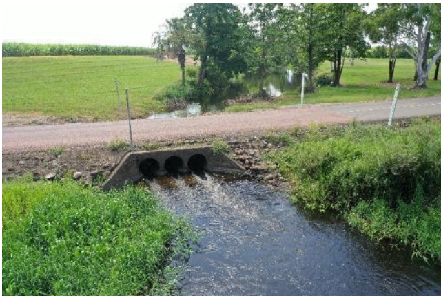
Photo 21. High flow velocities through the piped culvert of the Woodstock Giru Road crossing (above) present a fish passage barrier under most flow conditions short of road inundation. Increasing the height of the downstream discharge apron and reducing the flow slope and velocity through the culvert could provide an interim solution until the culvert can be upgraded to a more fish passage-friendly box culvert or bridge crossing.
