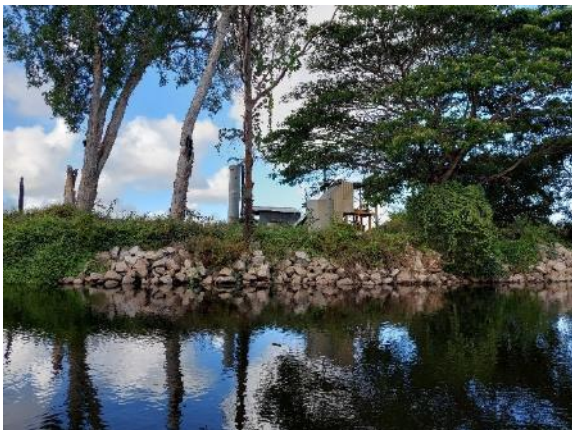
Photo 30. A lower lagoon reach that experiences high flow channel breakouts and associated erosion risks. Increasing the density of bank binding riparian trees at this site would serve to further stabilise the channel bank and baffle the velocity of outbreak flows.
