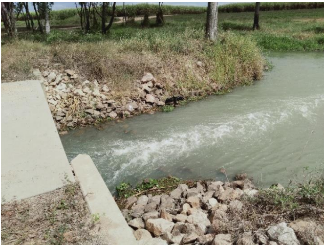
Photo 11. High flow velocities through road crossing culverts create fish passage barriers.
