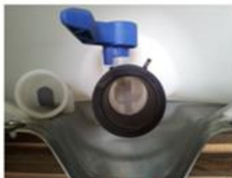
Water Tank Valve - OPEN
