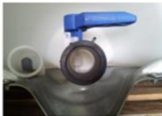
Water tank Valve - CLOSED
